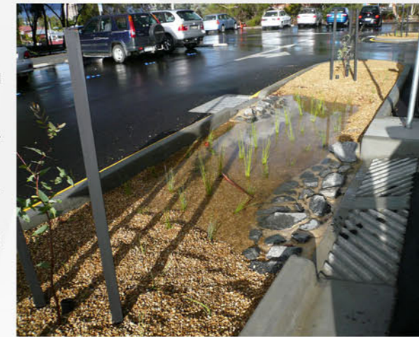
Car park bio filtration system
